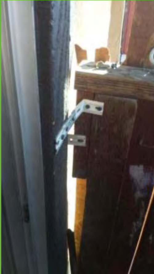
Improper balcony repair
