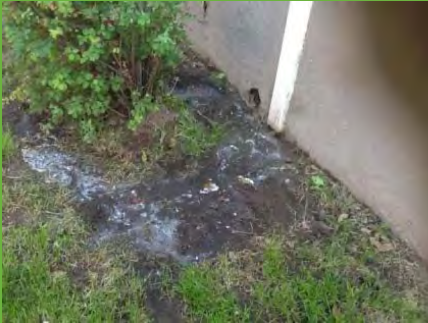
Raw sewage impacting common areas
