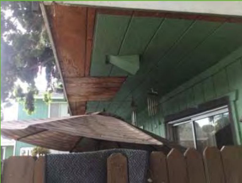
Unpermitted balcony repair
